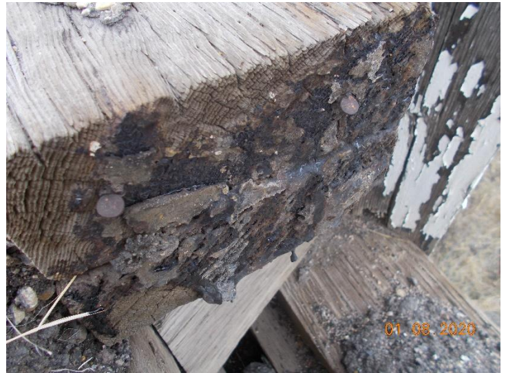
Suspect asbestos-containing material N-21-C-TR01. The black tar material is non-detect for asbestos.
